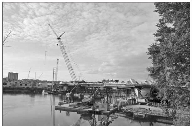
Construction continues on the Lowry Bridge. Pictured are views of recent work (from the east side looking north). Photos by Randy Klauk.
